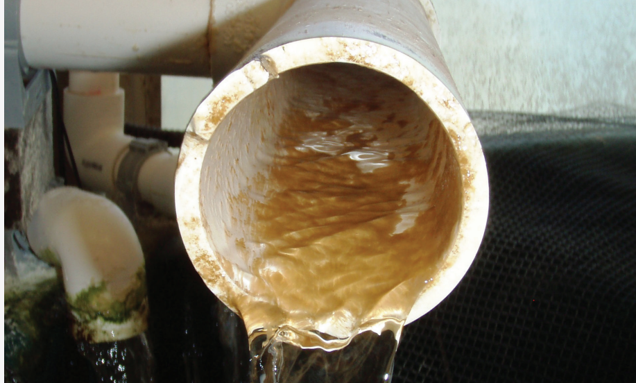
Figure 1: Pipe with a moderate biofilm.
